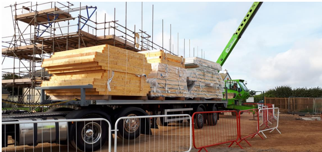
St Ann’s Chapel progress showing the start of the timber frame build process (photograph taken 17 September 2022)
